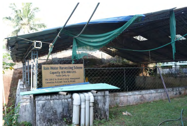
Rain Water Harvesting
